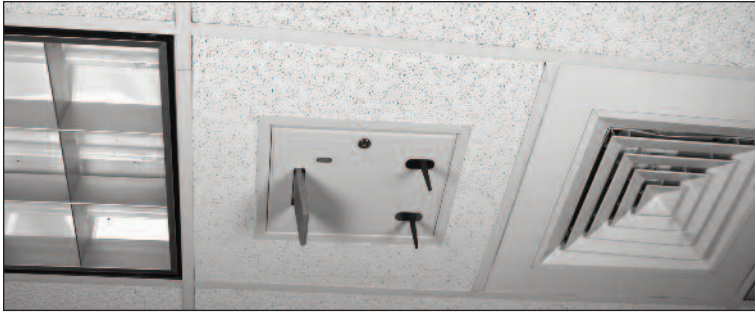
Application in an air handling space.
