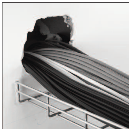
1. Existing hole with cables. Irregular hole cut.
