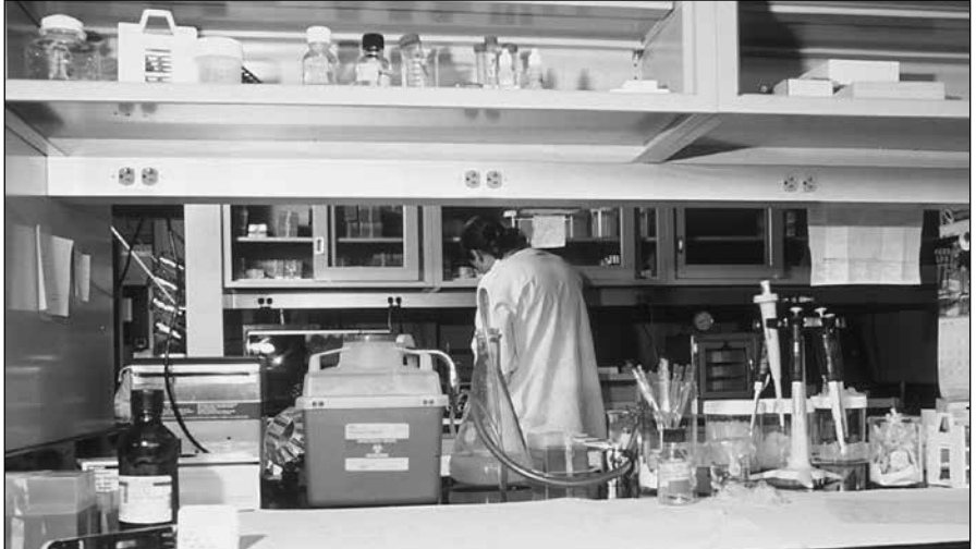
Standard devices installed in aluminum raceway mounted under reagent shelf in medical center lab.
