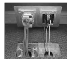
Flush activations offer a full range of power and communication connections.
